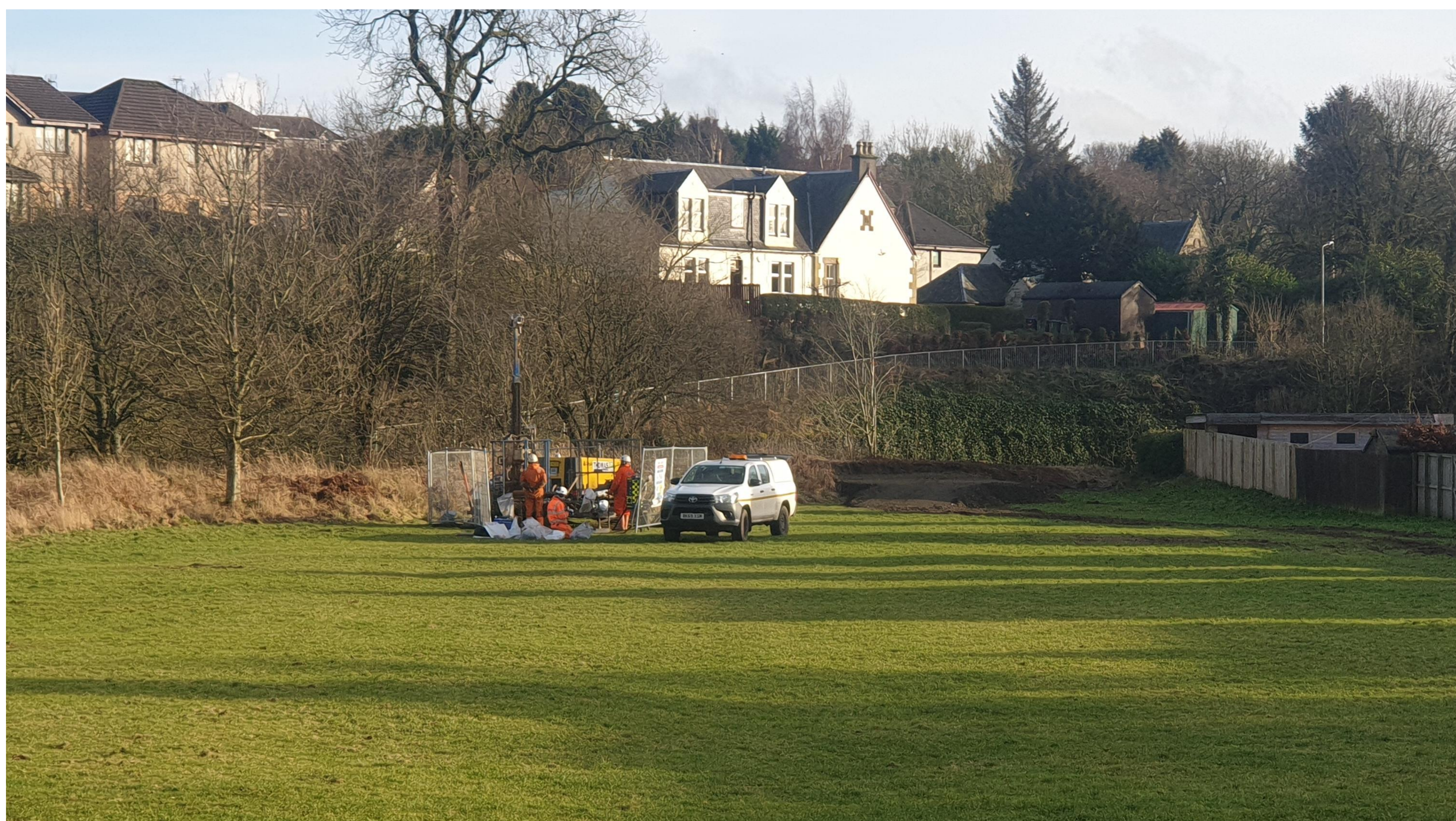
A bore hole drilling rig was used in Barbours Park in February 2024 to take a core of the rock strata to understand the ground conditions.
